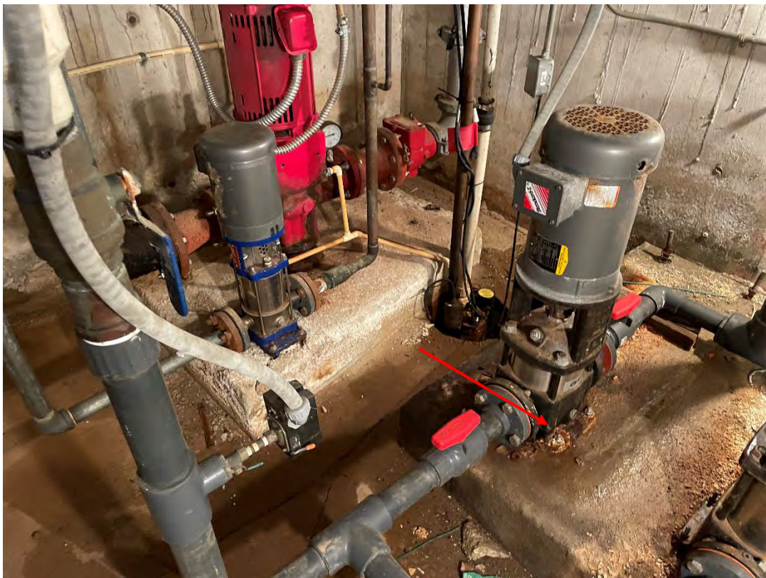
Figure 29 Pump room with corrosion on fasteners
