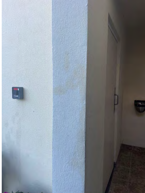
Figure 49A. Previous repairs with mismatched colors
