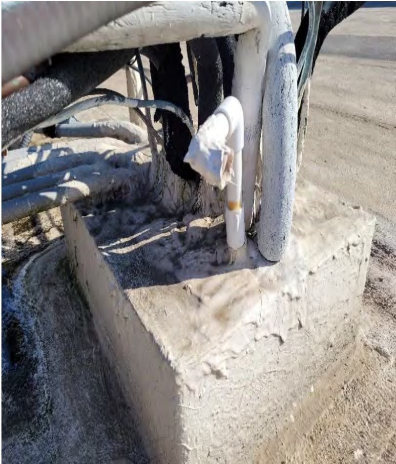
Figure 42 A/C mechanical equipment insulation showing deterioration
