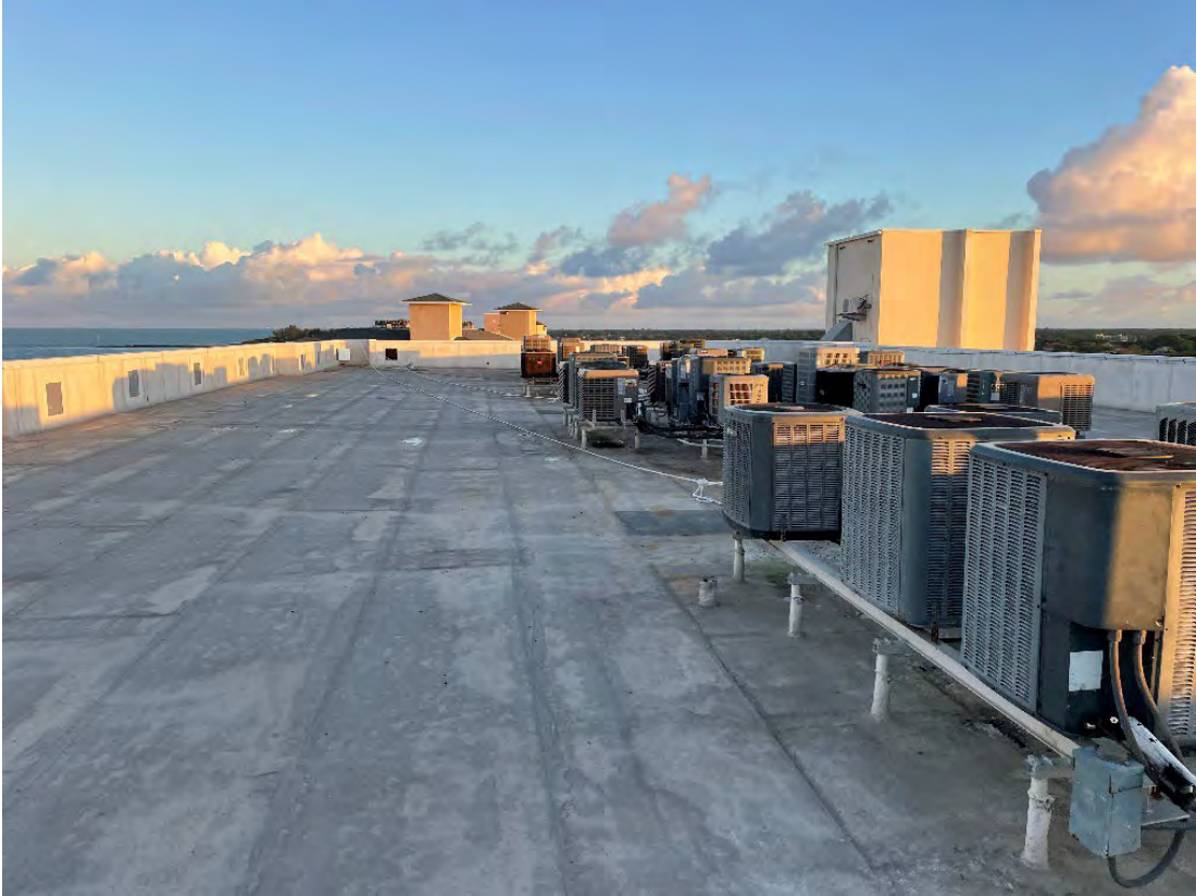
Figure 33 Modified Bitumen roof system with a roof coating applied
