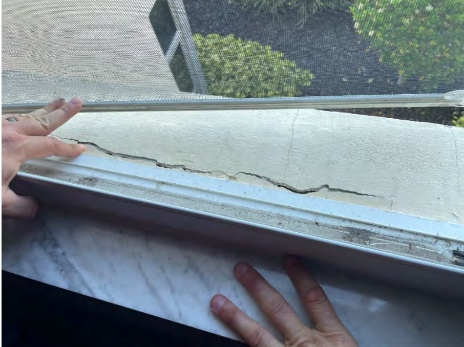
Figure 27 Typical Window Sill spalling
