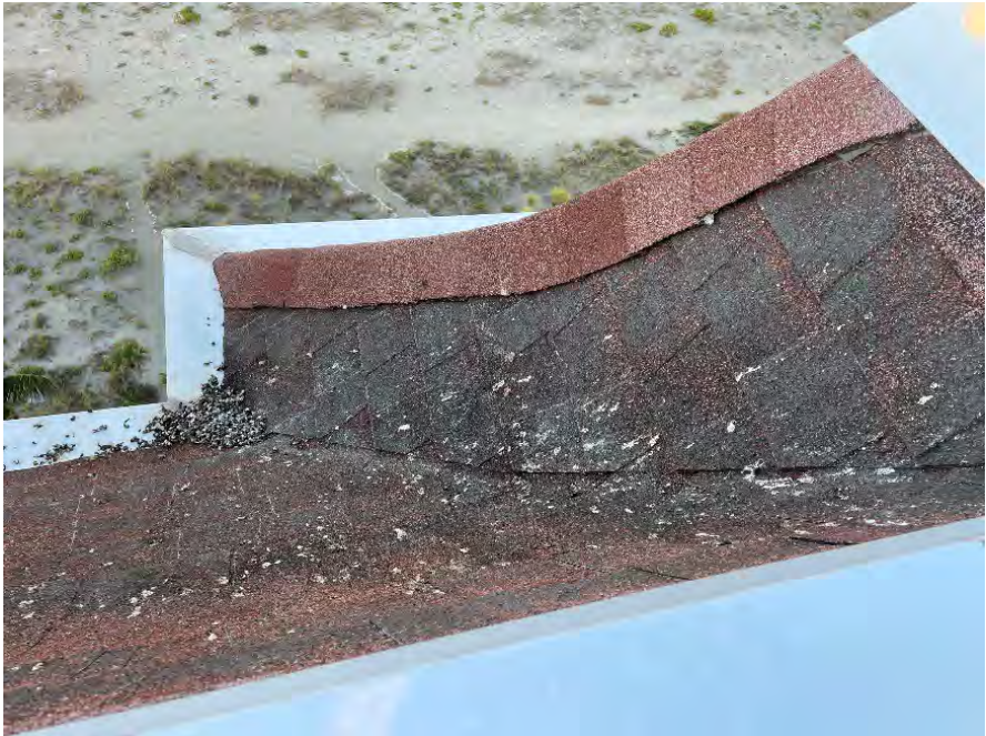
Figure 45 Organic growth on shingles
