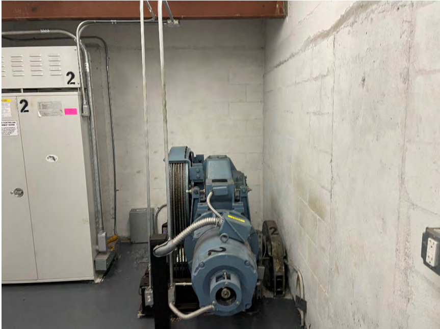
Figure 6 Elevator equipment room with CMU
