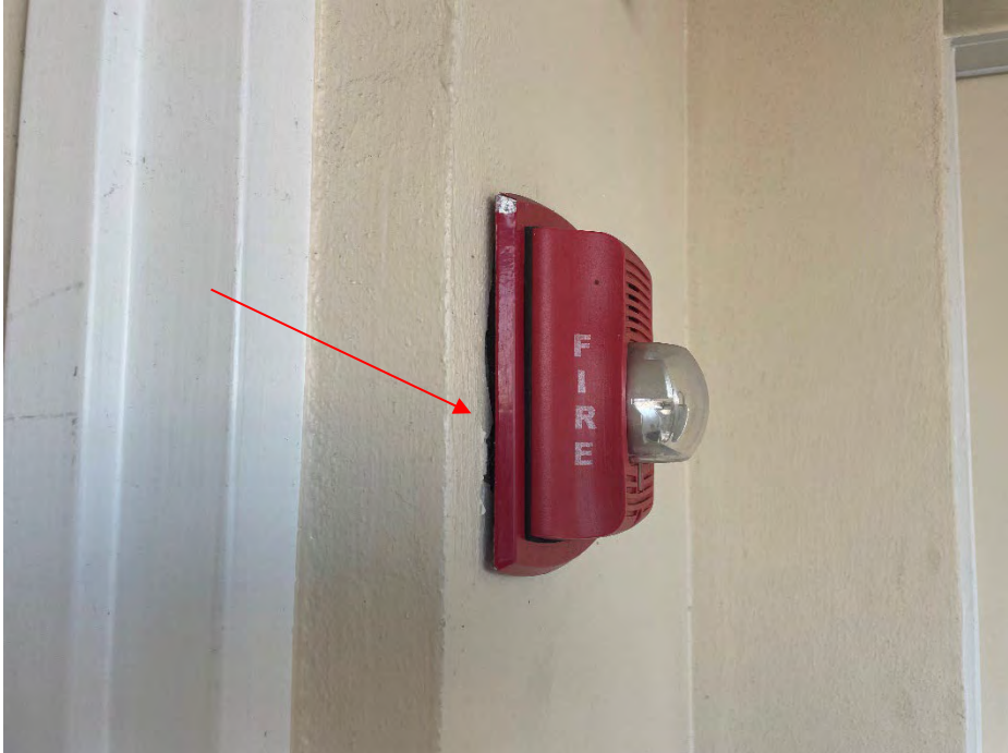
Figure 51. Protrusions lacking sealant
