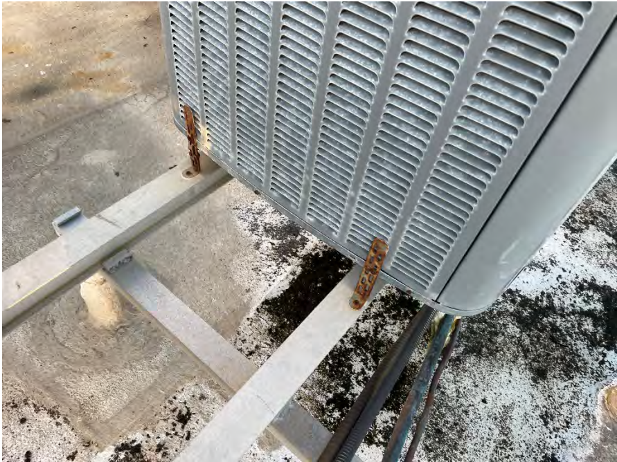
Figure 34 AC brackets appear corroded - owners responsibility to address as told to Karins by Gulf Shores
