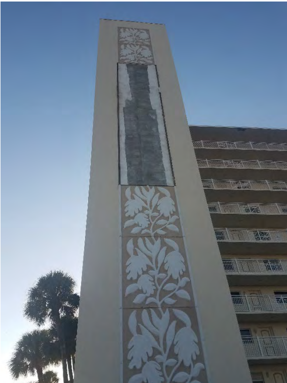
Figure 54B. Fiberglass decorative plates damaged from Hurricane Ian
