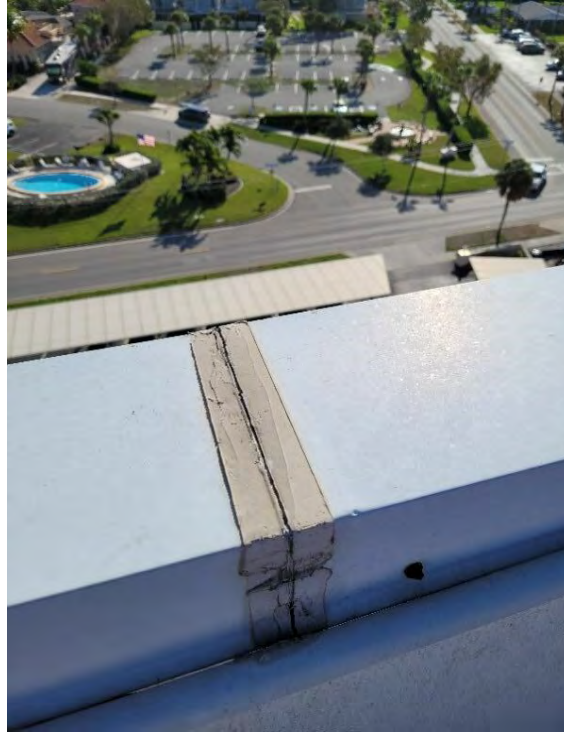
Figure 43 Recommend sealing coping seams
