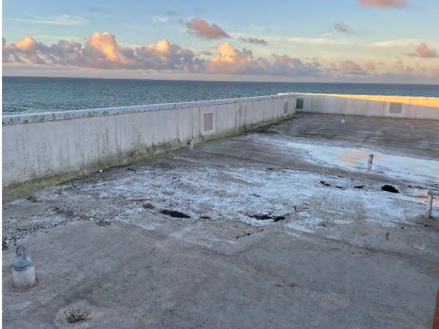
Figure 37 Roof appears dirty with residue from standing water
