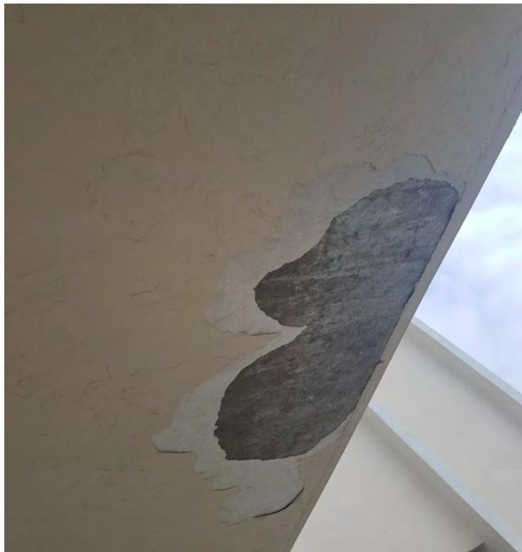
Figure 50B. Hurricane Ian stucco damage on 10 th floor
