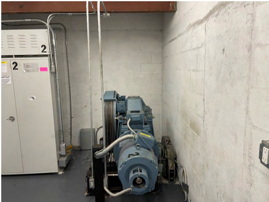
Figure 38 Traction elevator equipment room
