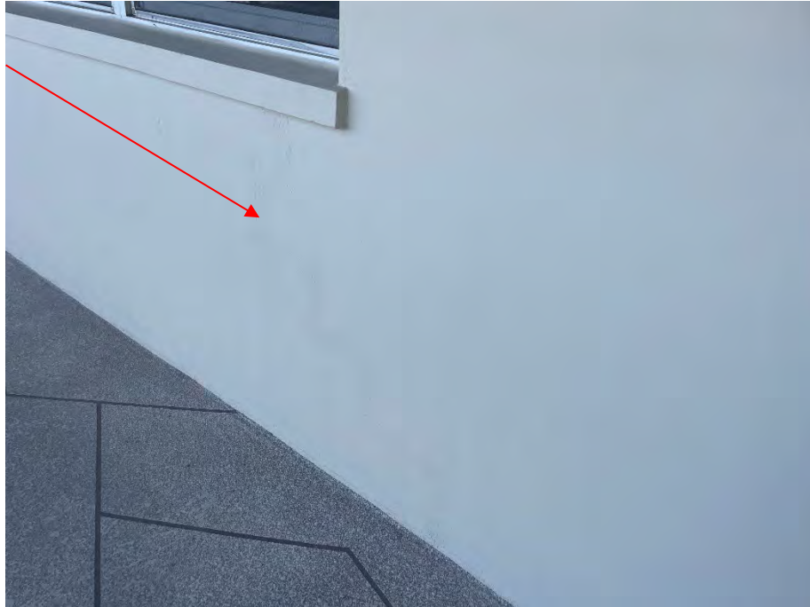
Figure 21 fine cracking at CMU at all elevations of walkways
