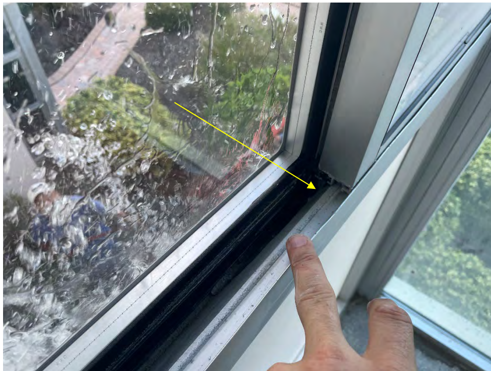
Figure 58 Areas lacking sealant may allow water into interiors
