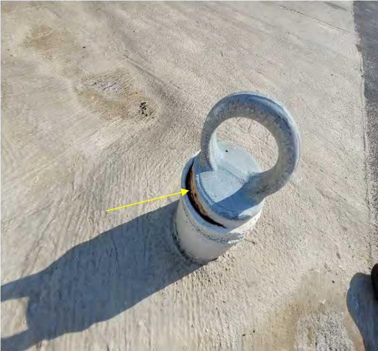
Figure 40 Open area at penetration to be sealed to prevent water intrusion
