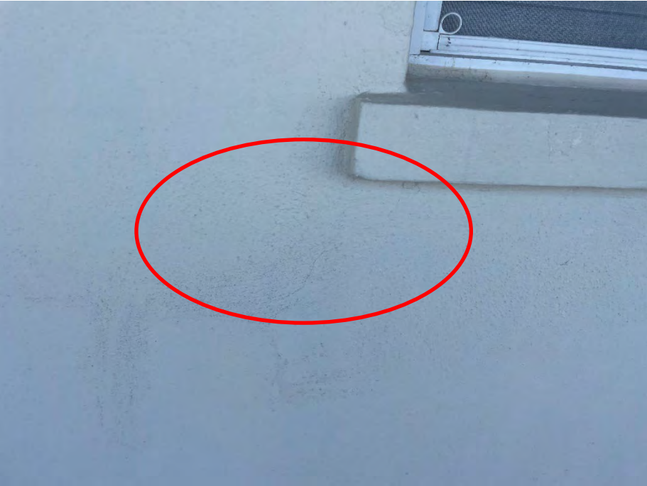
Figure 20 fine cracking at window sill
