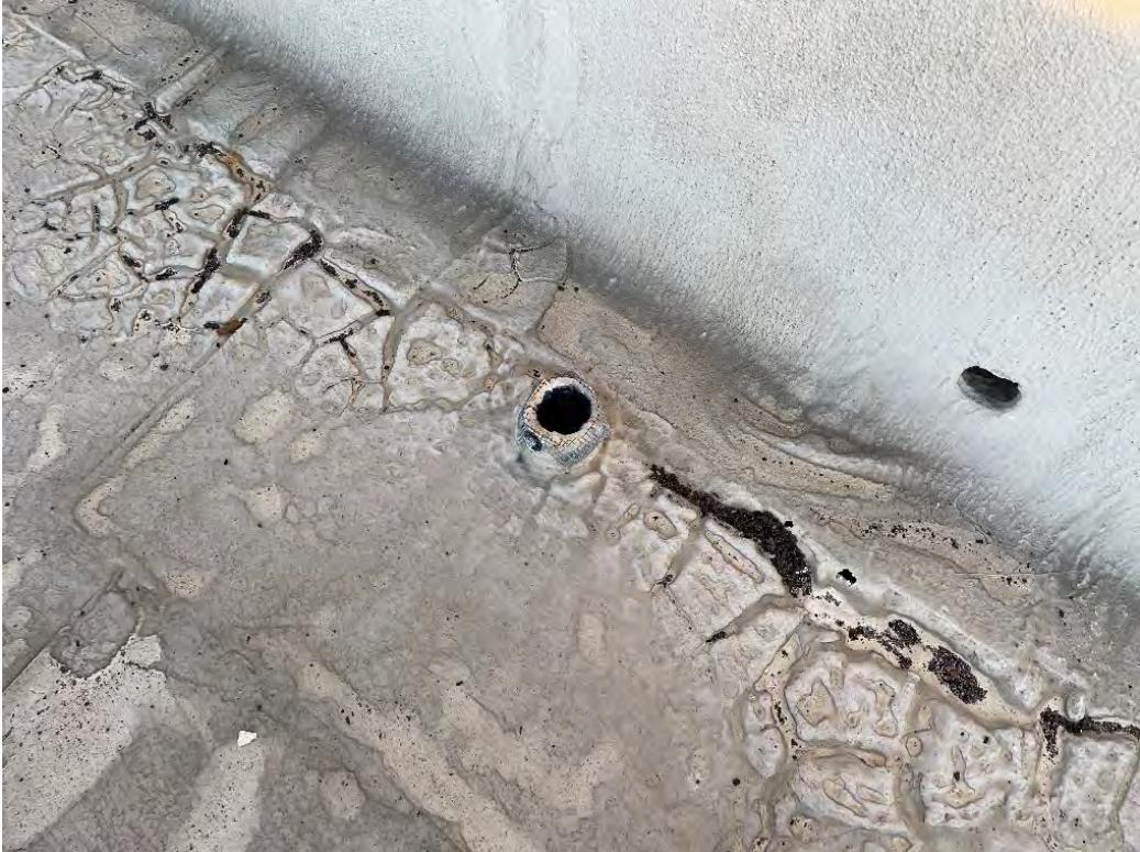
Figure 35 Roof Coating appears to be gatoring - roof membrane does not appear to be cracked
