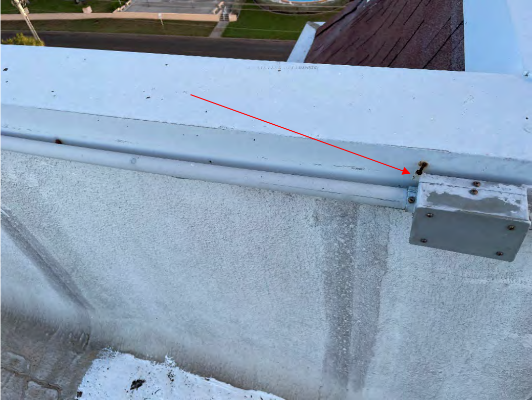
Figure 36 Loose fasteners are letting in water at coping flashing
