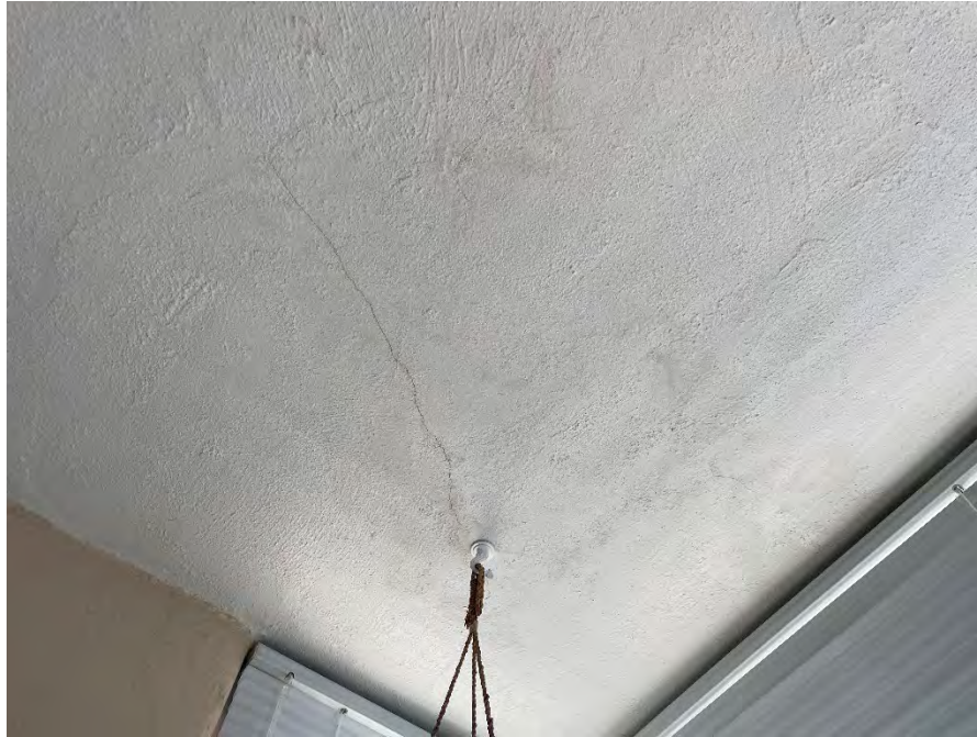
Figure 23 Balcony ceiling cracks observed at Unit 406
