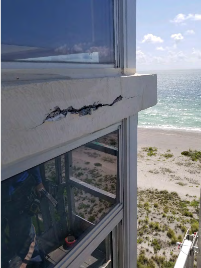
Figure 28 Spalling at slab edge
