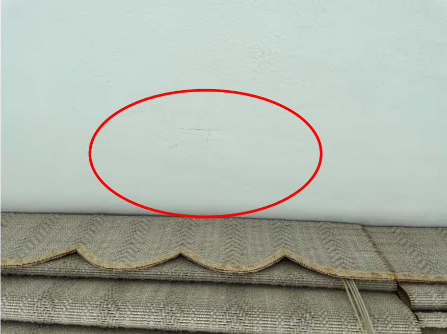
Figure 19 fine cracking at balcony ceiling
